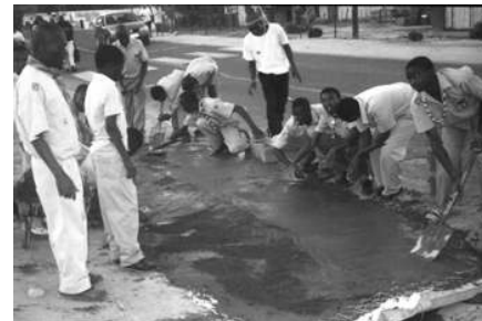
1st Sindzawonye Troop repairing the road entrance to the school, where the dip was too deep and cars were scraping on the verge. Troop Scouter Alfred Chirwa supervising the work with his Patrol Leaders..
